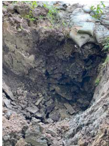
left finding the original draining sluices and then building the new clay wall on top of them
